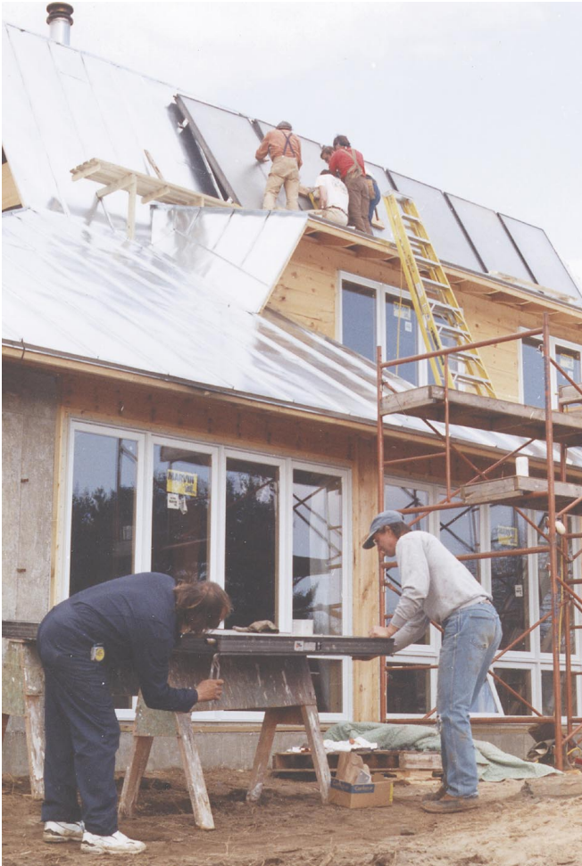
Above: The 4 x 8 panels are prepped on the ground, lifted to the solar ridge, bolted through the roof, and plumbed in place. A cat walk provides a good working platform and access for any maintenance.
